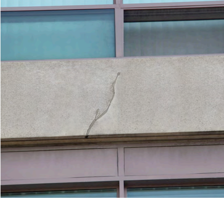
Figure 10: A fractured panel sealed to prevent water ingress. If a structural engineer assesses this panel to be safe, it will remain a visual issue but further damage can be mitigated by sealing the cracks, allowing for continued performance of the panel. Cleaning of the panel prior to sealing will greatly reduce the visual issues, but rarely totally eliminate them.
