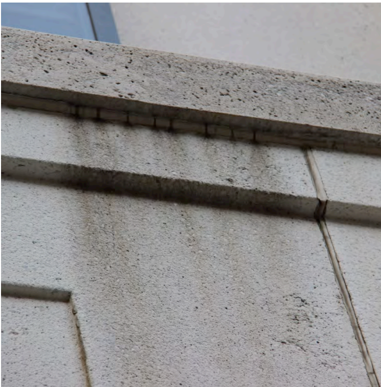
Figure 16: Drainage without weep holes. The horizontal sealant joint in the photo to the left is cracked and allows water to drain from underneath the window sill above. This is not a planned drainage path.
