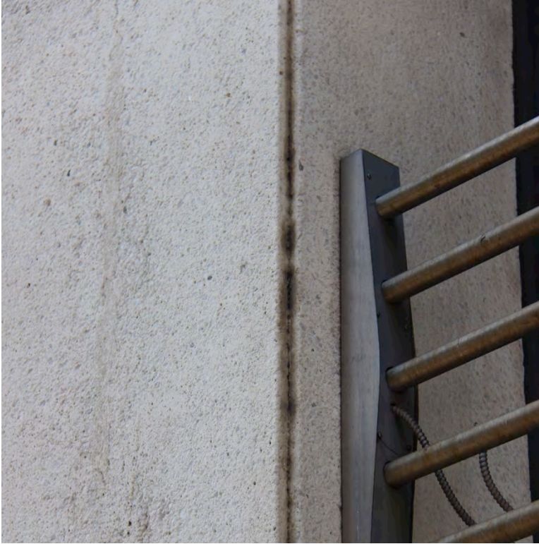
Figure 17: Attachments to precast panels may be structurally viable but, if the attachment points are not sealed to prevent water intrusion, this could lead to cracking of the precast panel.
